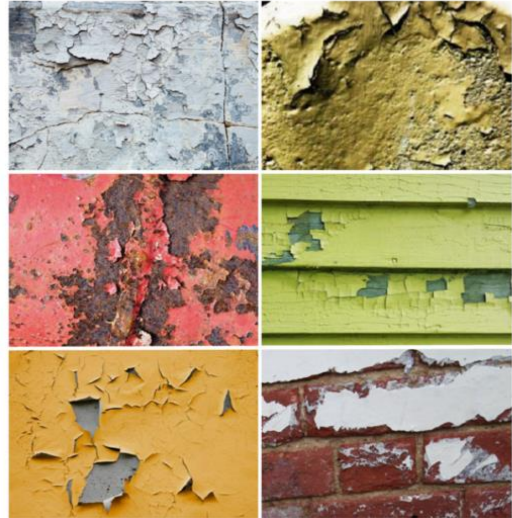
Figure 1. Deterioration of architectonic coatings
